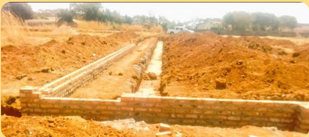
Construction of Nharira School, Norton only commenced after ZACC intervention through a compliance spot-check exercise
